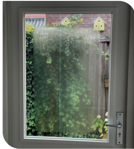
Condensation on the interior side of the glass.
